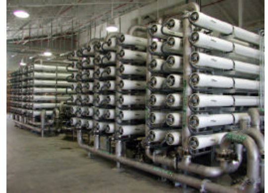
Above: Alameda County Water District's Brackish Water Desalination facility
